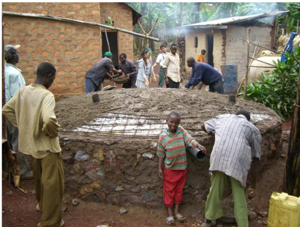
Village inhabitants and members of the organisation Ingenieure ohne Grenzen e.V. are working hand in hand on the cistern project.
